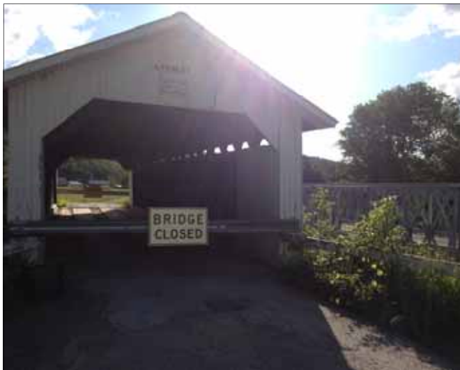
Figure 47. Photograph of the current condition of the Longley Bridge, Montgomery, VT. Photo by Shana Stewart Deeds
