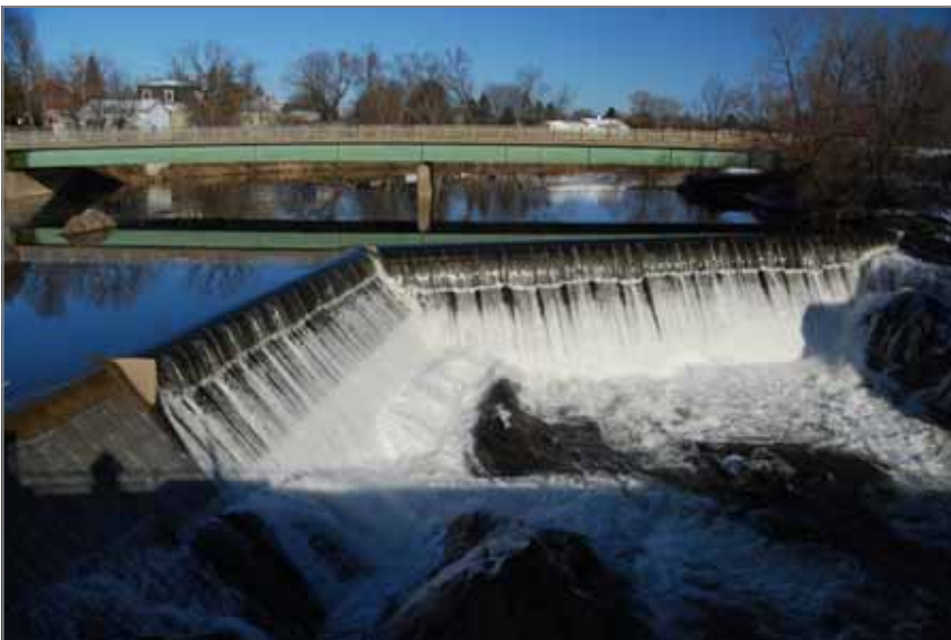
40. The dam and falls at Enosburg Falls, taken from the historic Bridge of Flowers and Light (photo by Shana Stewart Deeds).
